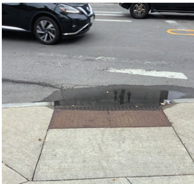
Caption: Curb ramps with ponding.
